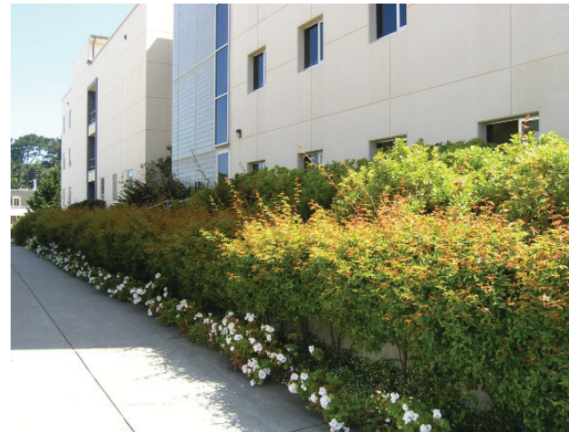
Overgrown shrub planting needs trimming or replacement.
