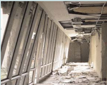
Northridge Earthquake, Los Angeles Area, 1994
