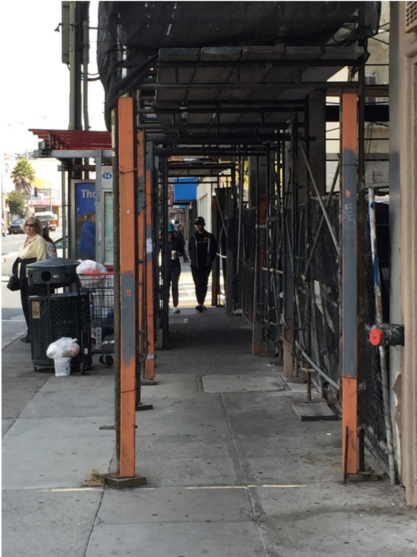
Bus Shelter on Mission near Russia, in conjunction with construction (long term) leaves very little room for pedestrians to pass by safely.
